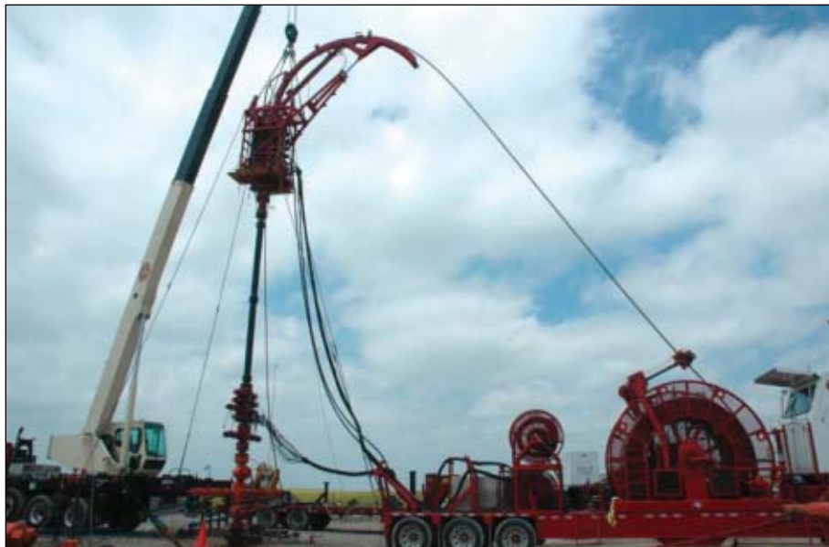
A CT unit from Bobcat Pressure Control Inc. works on a Barnett shale well in May on the Walsh Ranch, west of Fort Worth (Fig. 4, photo by Nina M. Rach).
